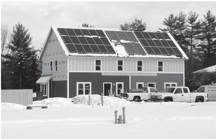
Exterior view of two Wisdom Way units under construction this winter. photo by Anne Perkins
