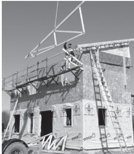
Truss being lifted into place on the second of four Habitat for Humanity Houses designed by Kuhn Riddle photo by Erika Zekos Assoc. AIA
