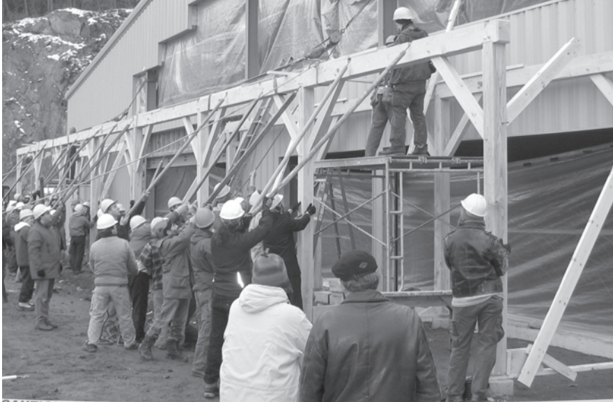
Volunteers raising the timber frame at River Valley Market photo by Suzanne Webber
